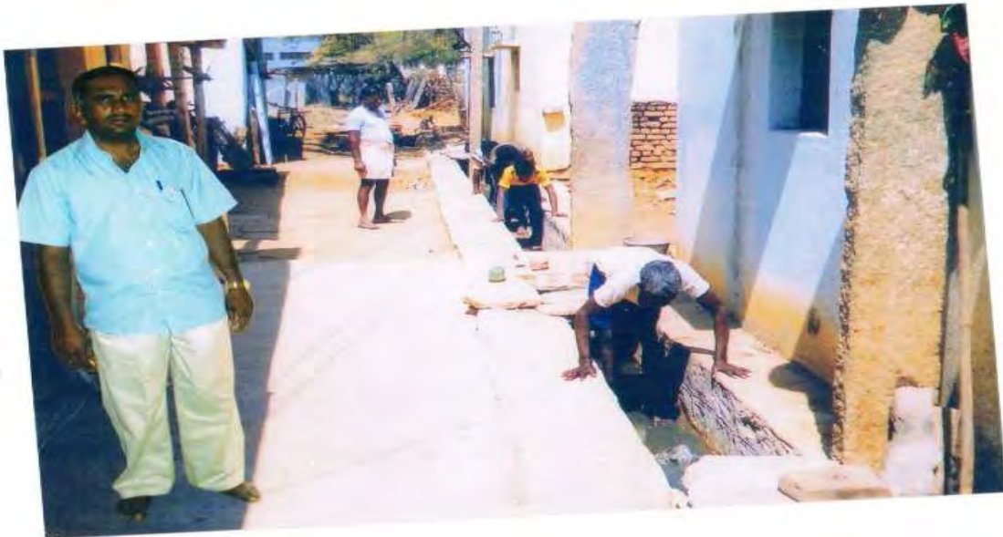
Under a complaint made by a citizen in J Thammasandra in Kolar, the drains are seen being cleared.
